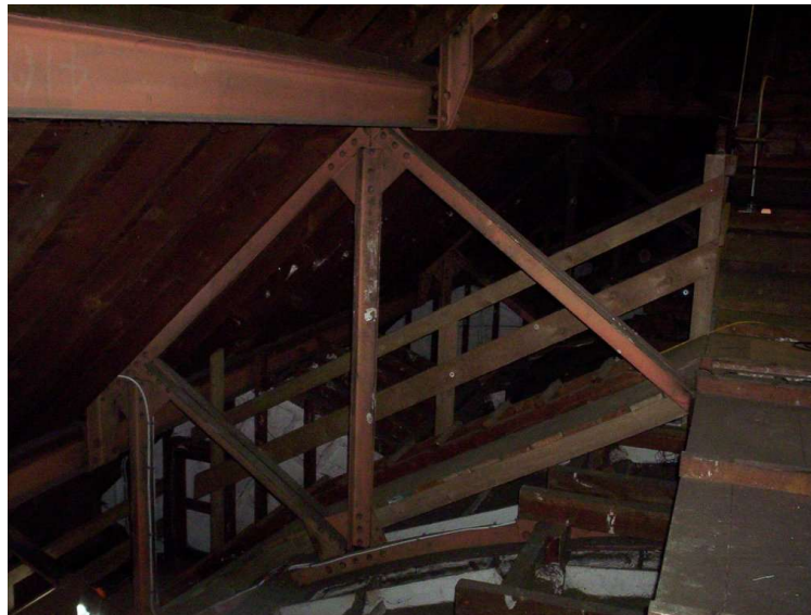
Figure 10: Photograph of the interior of the roof void in the Great Hall from previous audit work by contractors showing no obvious insulation
